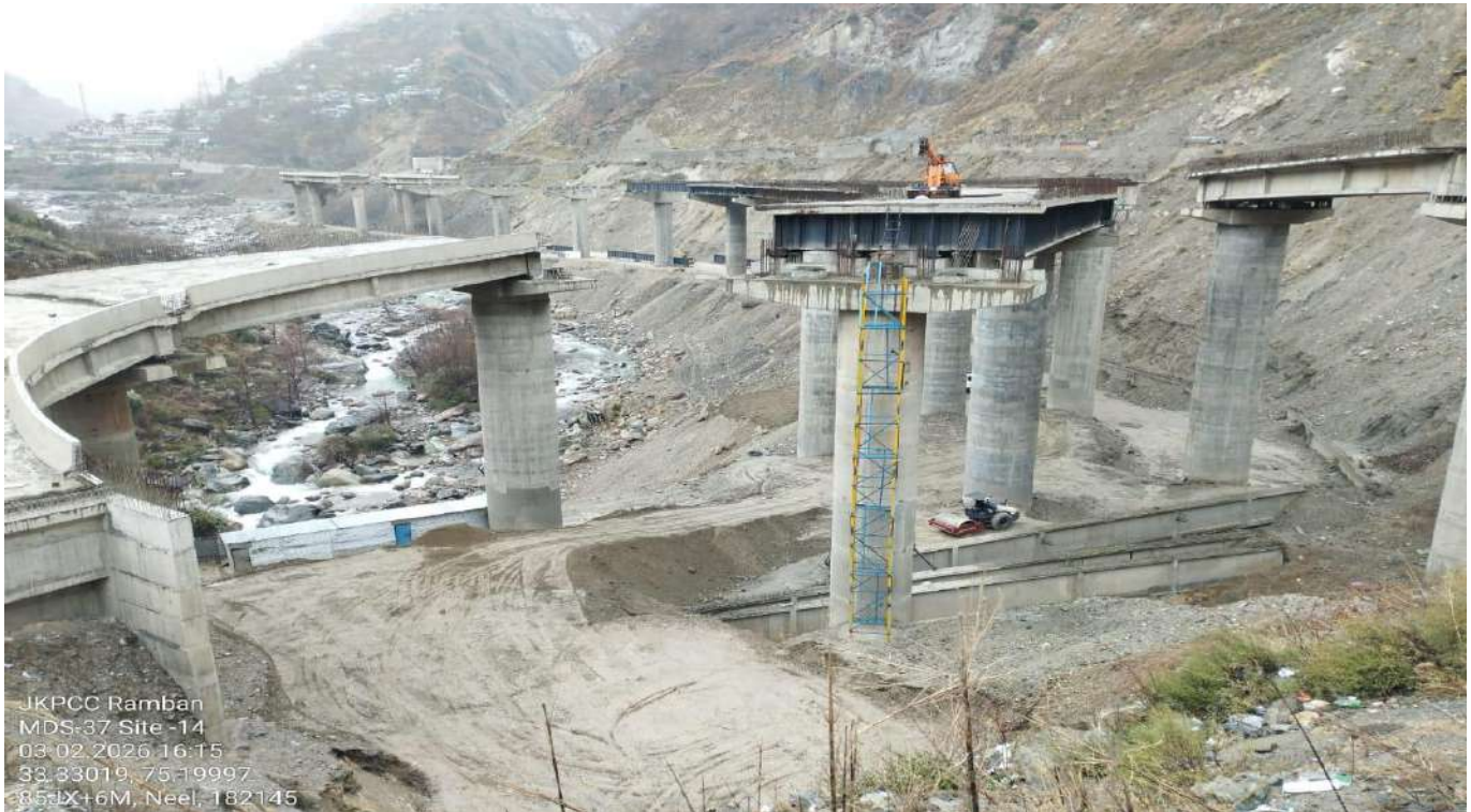
The toe production work needs to be done on completion of viaduct work.
