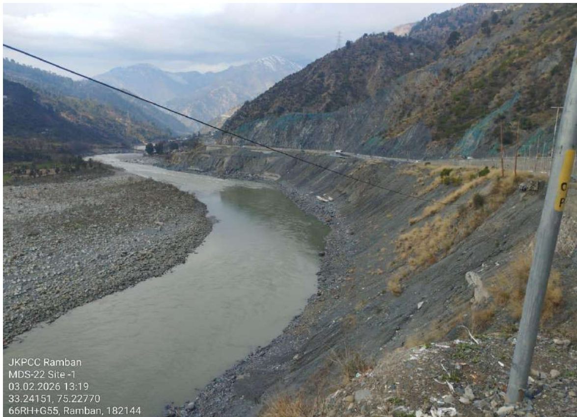
Gabion at bottom washed away due to recent floods but slope is stabilized and closed.
